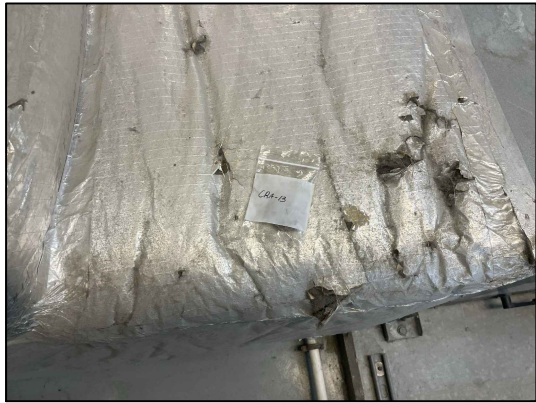
15. View of non-ACM containing duct insulation sample CRA-13 located in the women's side maintenance room.
